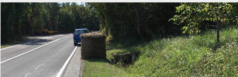
Concrete drain not protected
