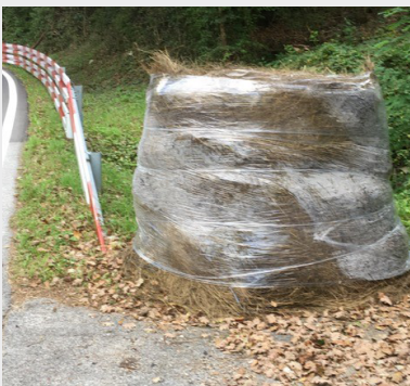
Guardrail nose not protected
